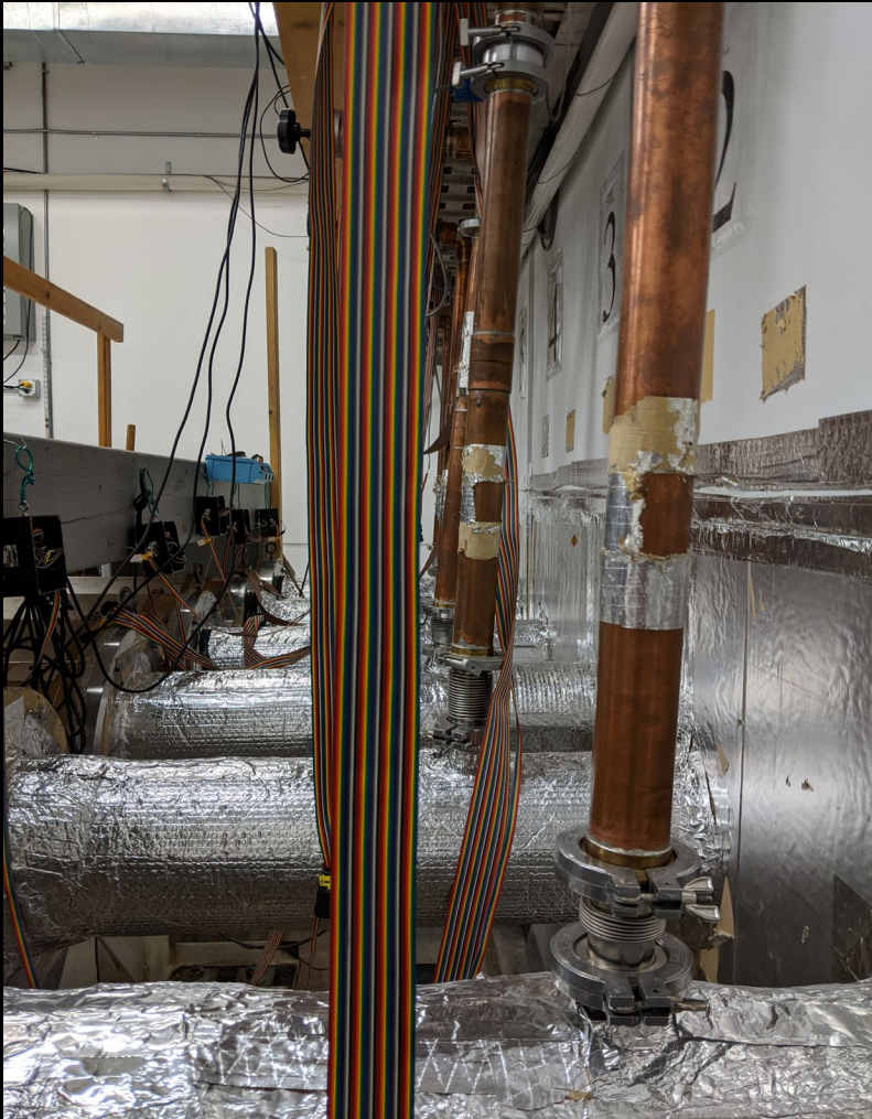
Image: Connection of snouts to manifold
