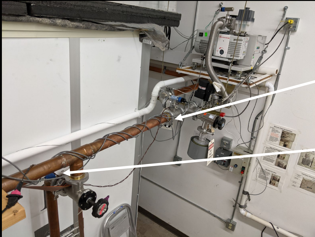
Image: Pump and current vacuum lines
